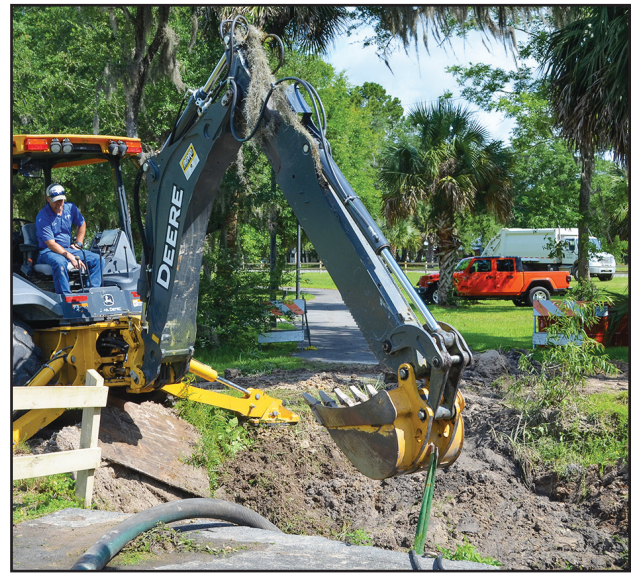
City crews were busy digging up the box culvert Thursday to determine if it can be repaired or must be re-built.
